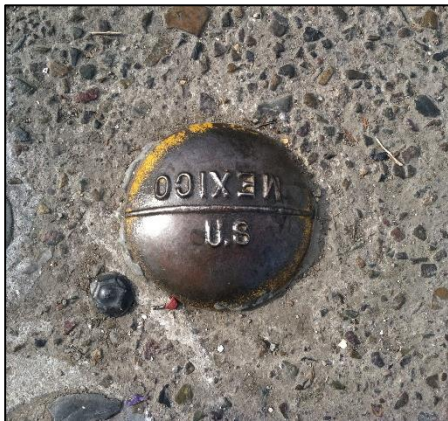
U.S./Mexico border delineator in the pavement at the San Ysidro/Puerta México-El Chaparral POE
