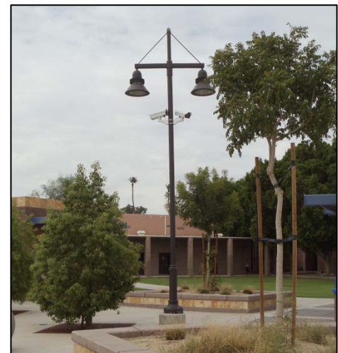
Bus stop lighting and security cameras
