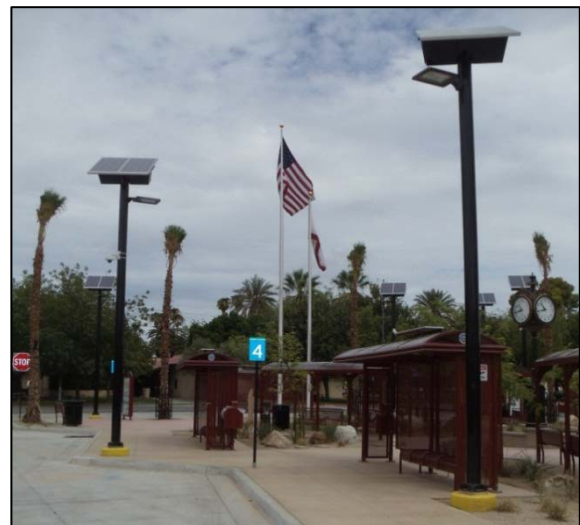
Typical transfer station lighting
