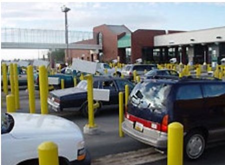
Typical license plate reader installation
